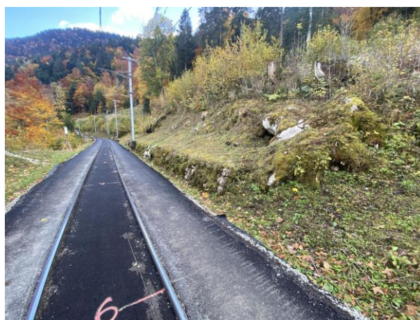
Figure 22 : KM 25.100 – Mur amont
